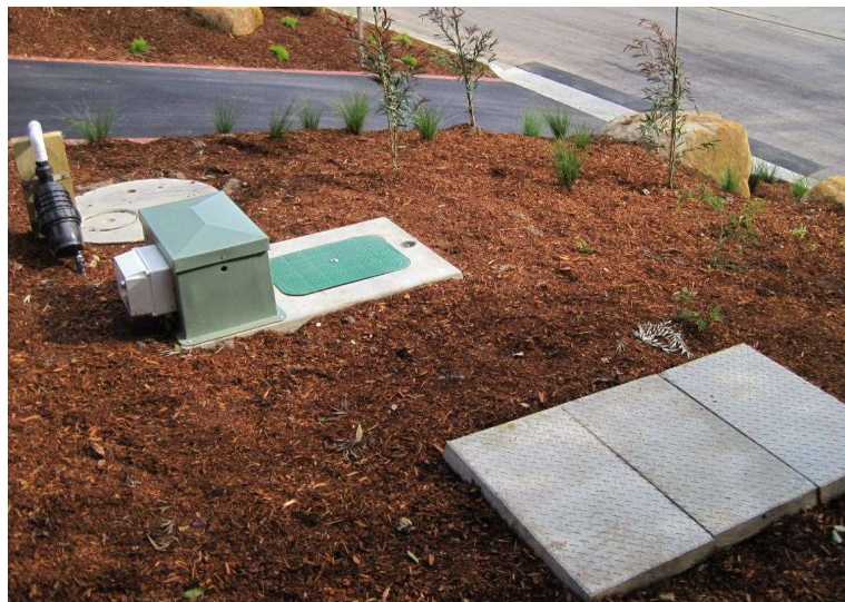
Figure 2: Treatment Plant with sub-surface irrigation
