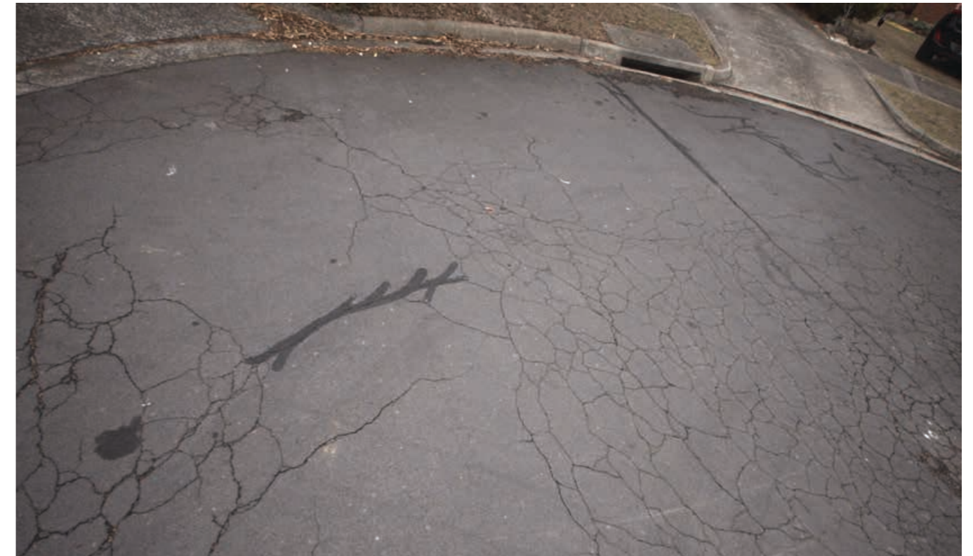
Figure 19 Snapshot of a very poor road surface (Wallmah Close in Templestowe)
