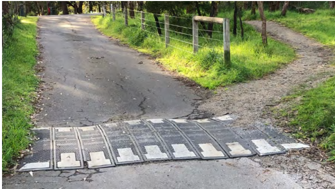
Image provided by a local resident regarding the speed hump
