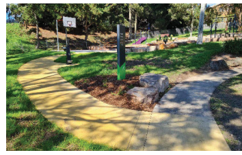
Brendan Reserve Playspace Renewal completed including new ball court, access path, furniture, and landscaping
