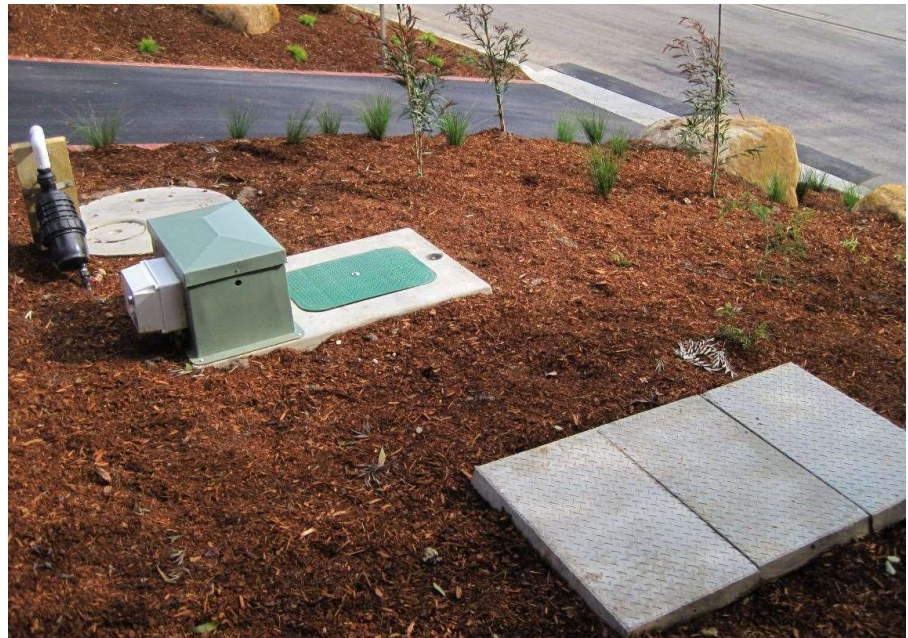
Figure 2: Treatment Plant with sub-surface irrigation
